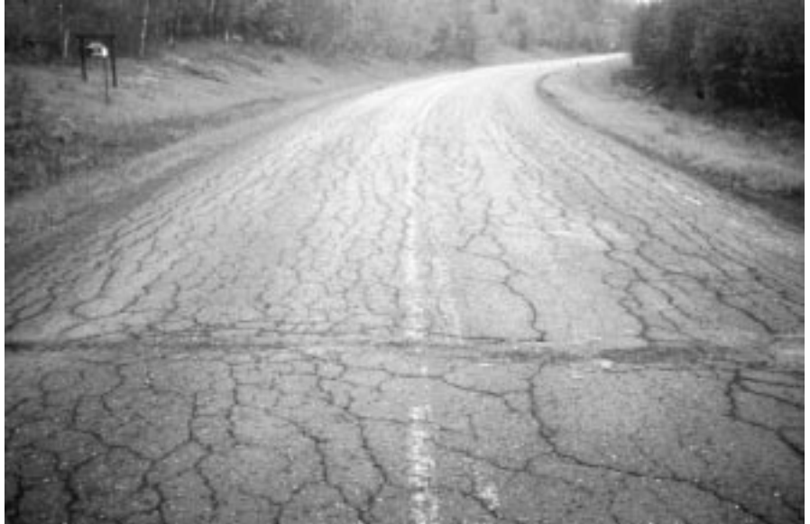
▶ Extensive alligator cracking. Pulverize and rebuild.
