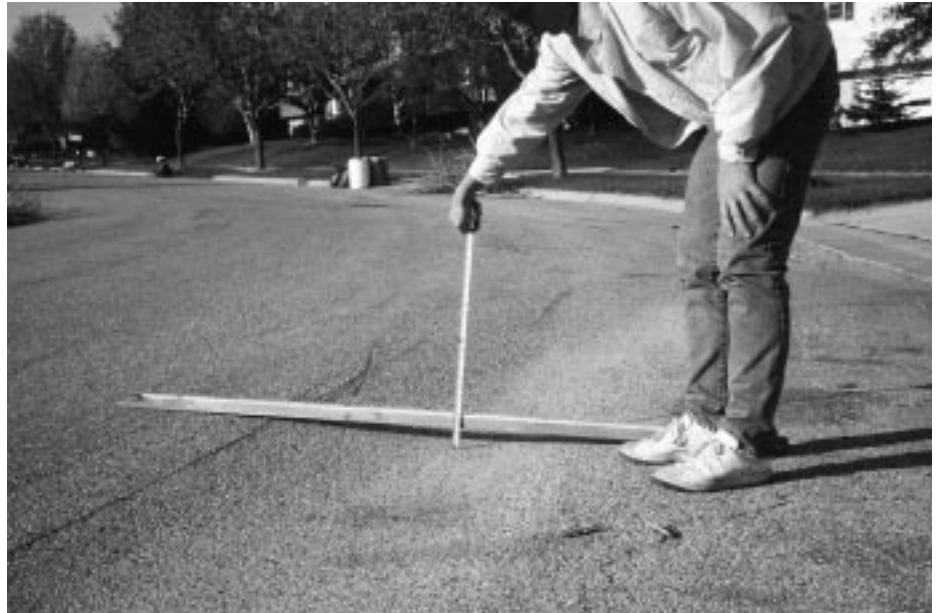
► Severe settling from utility trench.
