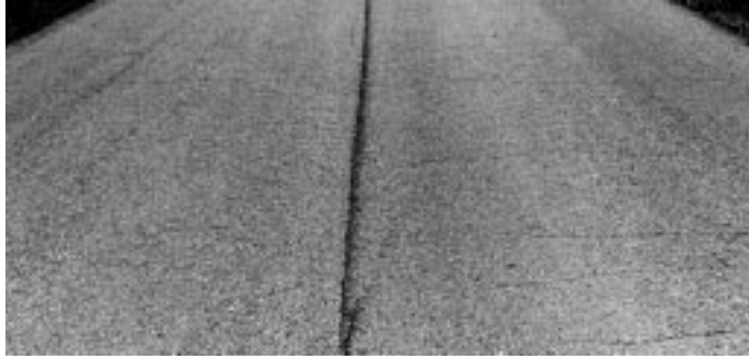
Centerline crack (still tight). ▶
