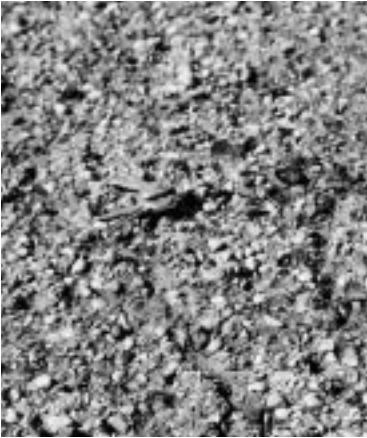
Severe raveling with ▼ extreme loss of aggregate.
