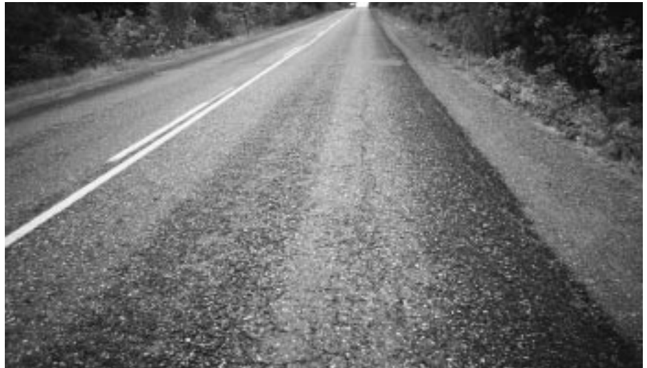
► Moderate to severe raveling in wheel paths.
