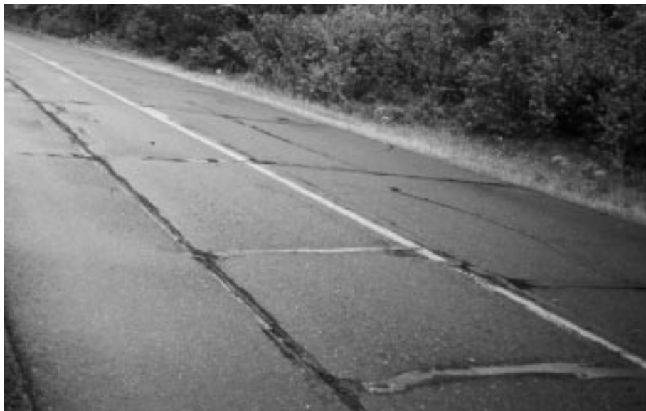
► Concrete joints reflected through bituminous overlay.
