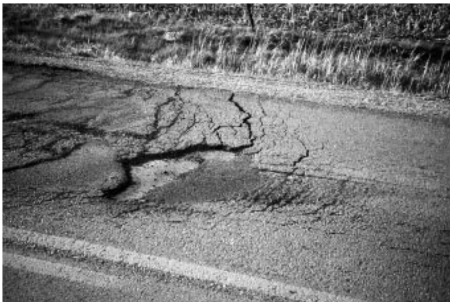
► Loss of bond between pavement layers allows traffic to break loose pieces of surface.
