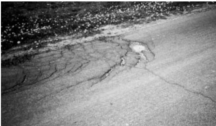
► Crescent-shaped cracks characteristic of slippage.
