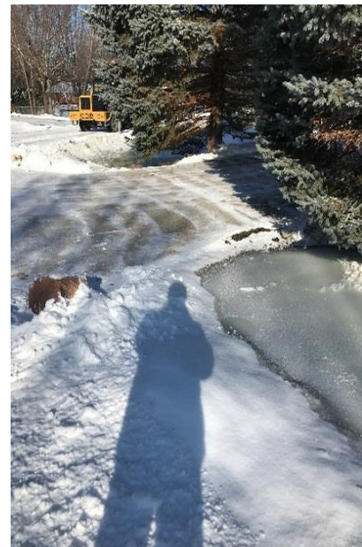
Figure 1. N178 Van Handel Drive (Ditch Full, Culvert Pipe Not Visible)
