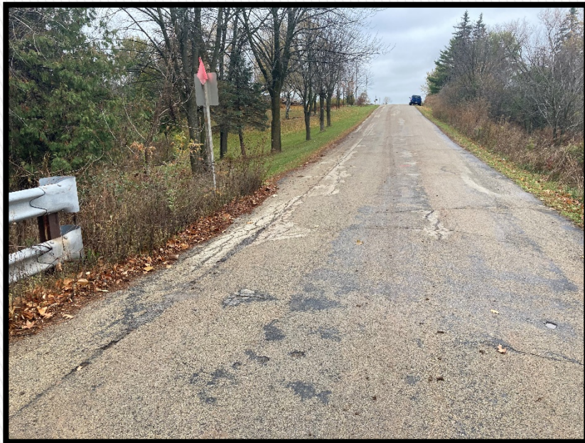
Deck has been patched and overlaid with asphalt (looking north)
