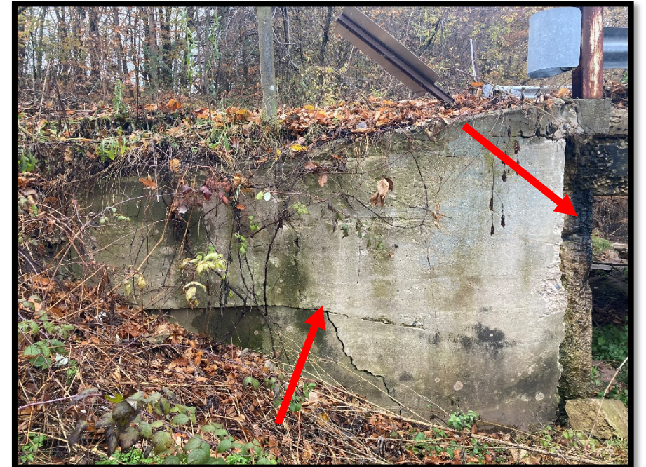
Wings are failing and are severely cracked
