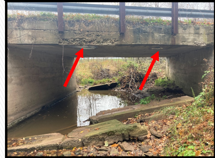
Exposed gravel (spalling) and rebar along deck edges
