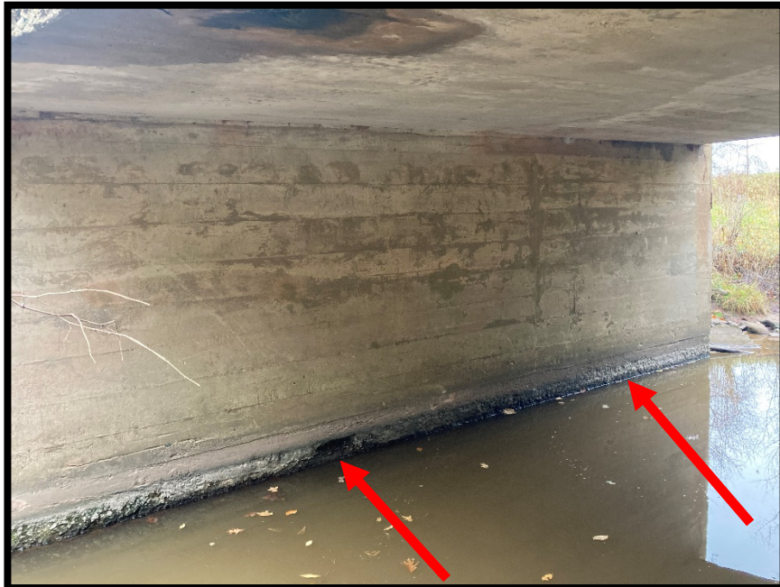
Scouring has deteriorated the base of the abutments.
